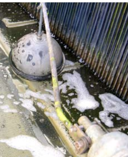
Regularly check level of cooling tower
