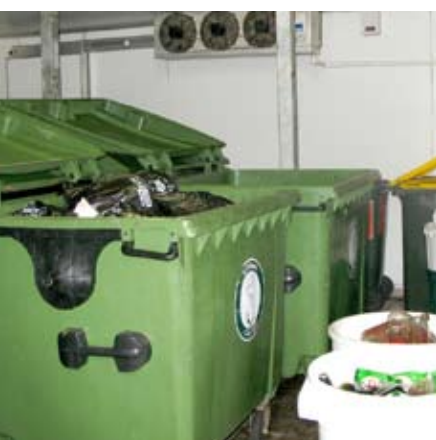
Storage of waste in a cool room at Sirromet Winery.
