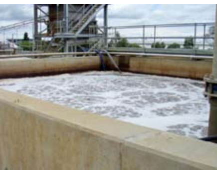
Wastewater treatment systems can be a source of odour if not operated correctly.
