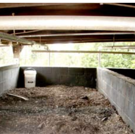
Enclosed biofilter at the Australian County Choice processing plant.
