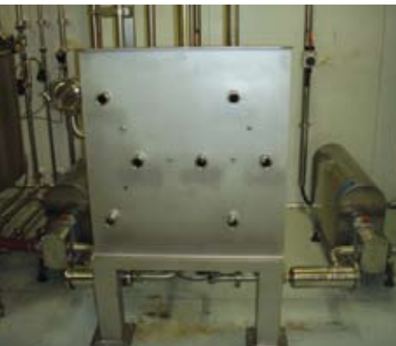
CIP systems can save labour, water, chemicals and money.
